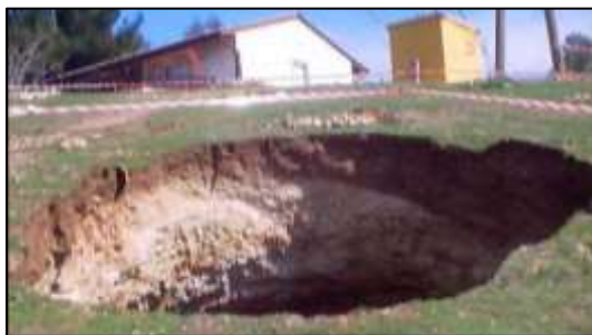
Figure 3. A Recent Developed Sinkhole (Down-Stream) After Filling of the Reservoir (Al-Ansari et al. , 2015b).
